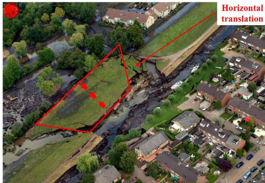
Figure 3 Horizontal Failure of Wilnis Levee, occurring in 2003 after a drought (image courtesy of Prof. Stefan Van Baars).
